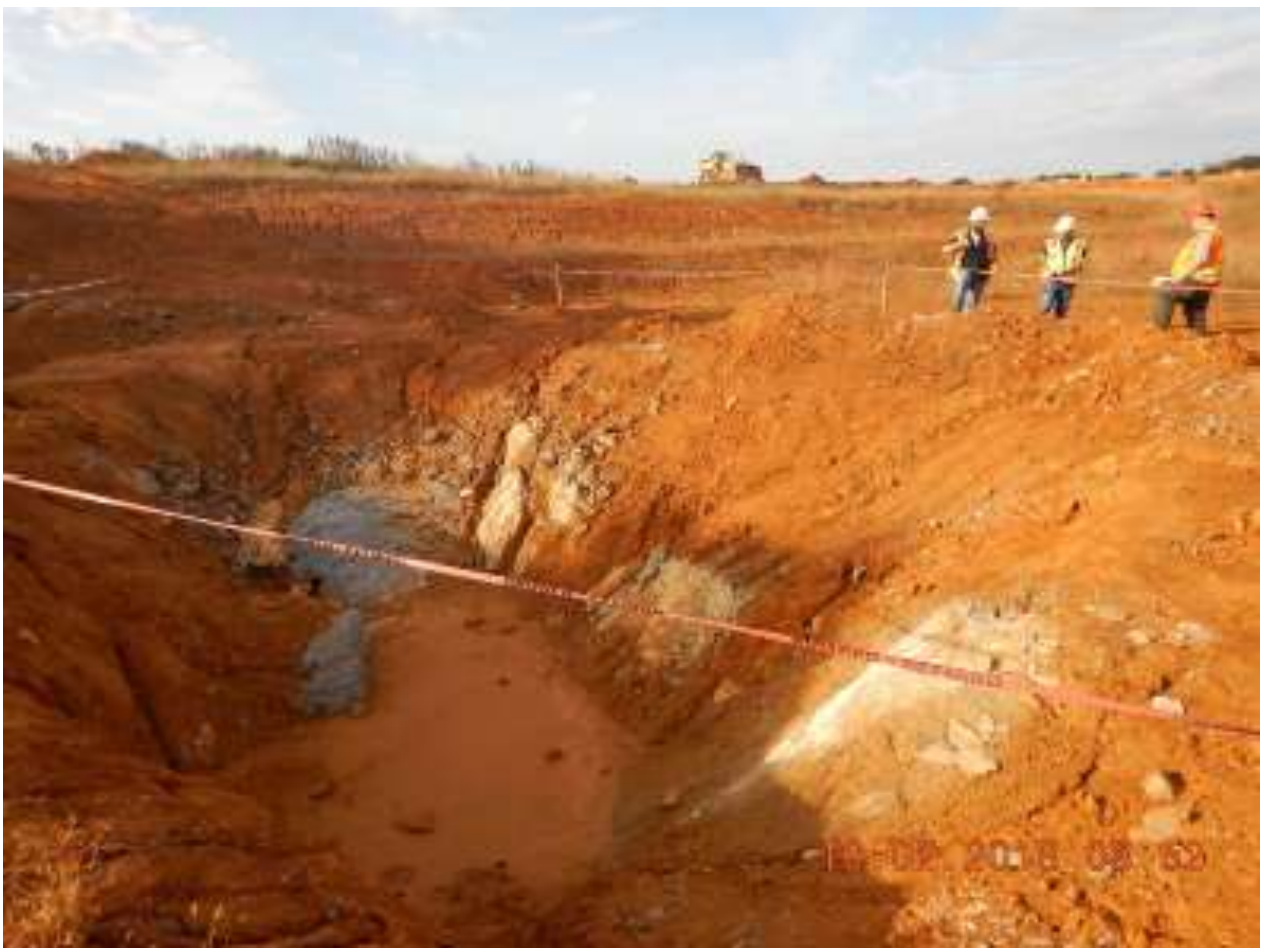
Sinkhole in Basin #1
