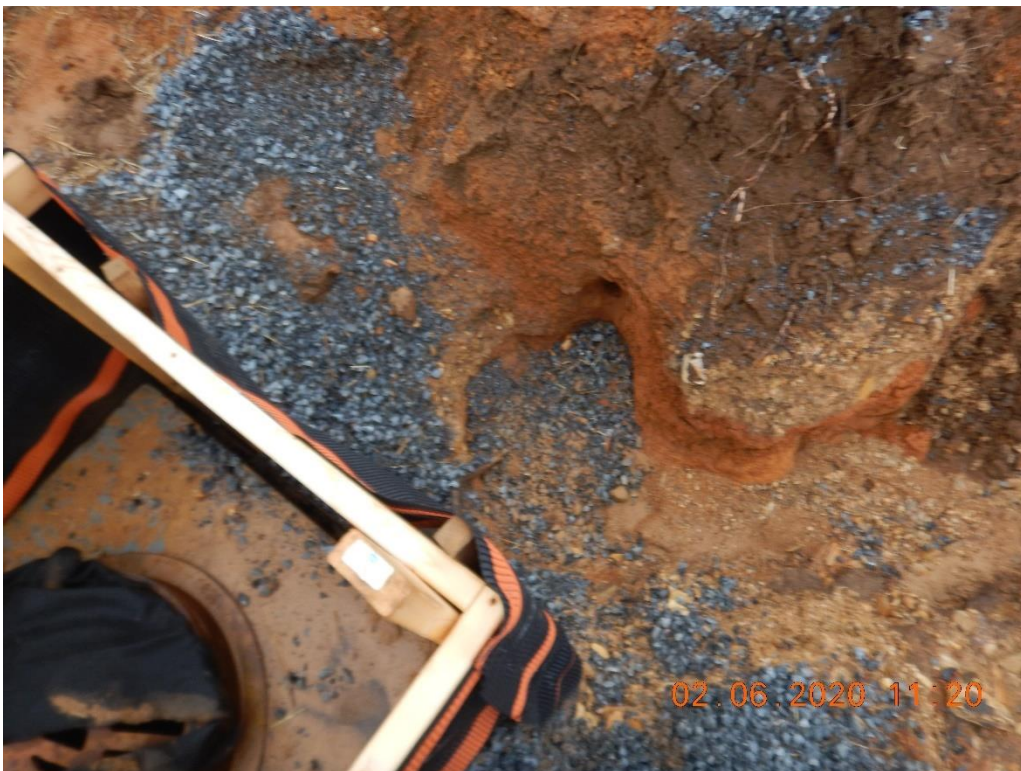
Maintenance on Drop Inlet protection where rock apron has been eroded away.
