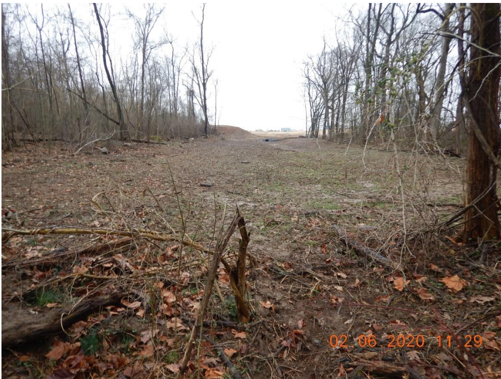
Diversion channel #1 and rip rap apron #2 not installed at time of inspection.
