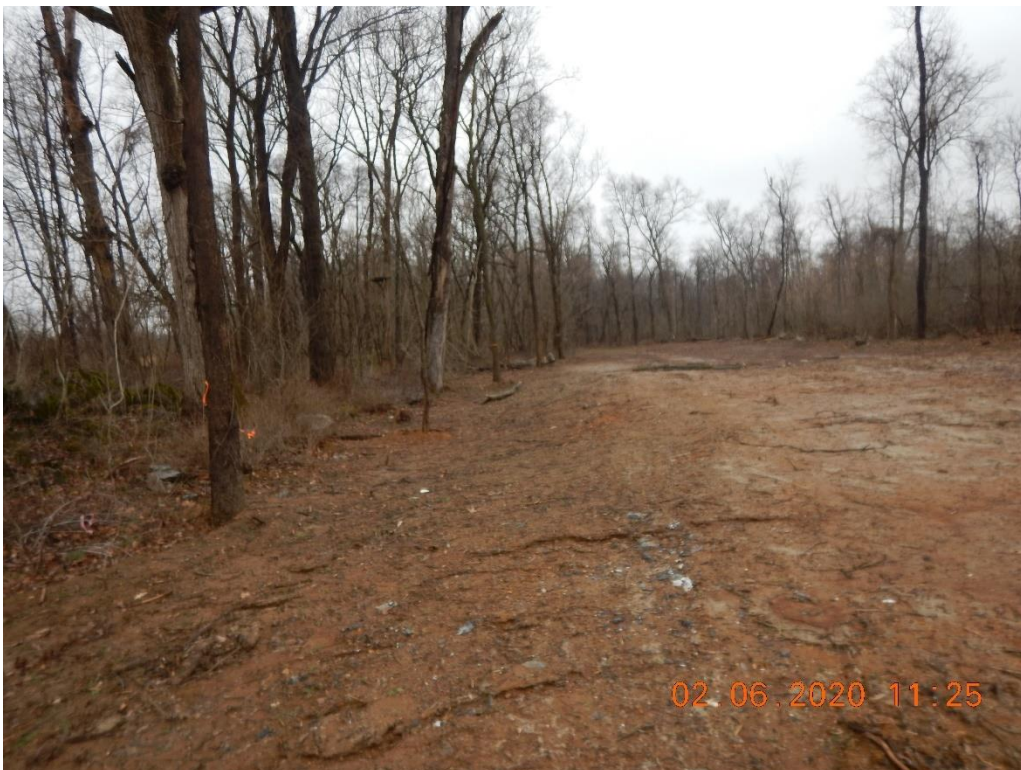
No perimeter controls installed along LOD along collection ditch #1.
