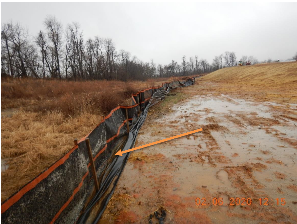
By-pass under silt fence that allows sediment laden water to leave the site.
