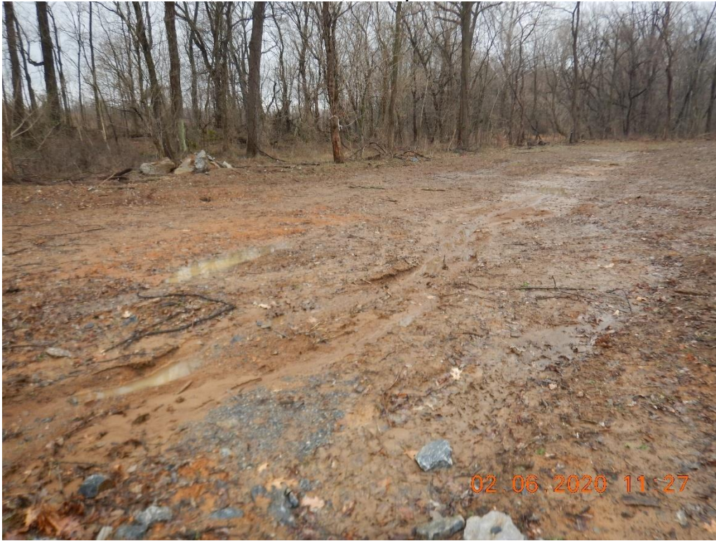
Diversion channel #1 from sediment basin outlet not installed.
