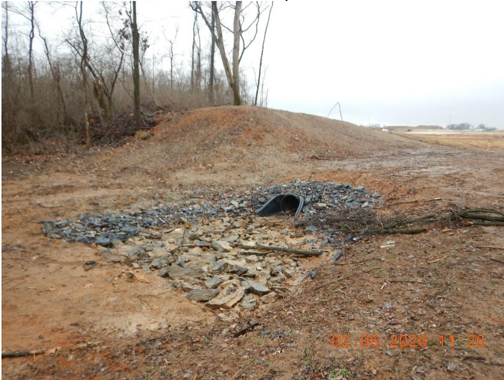
Outfall of sediment basin with not signage posited. Rip rap apron is stained with sediment from improperly operated basin.
