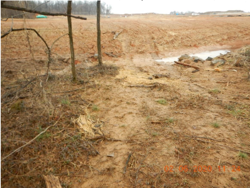
Sediment deposit outside the LOD below Sediment Basin. No perimeter controls installed at this location.
