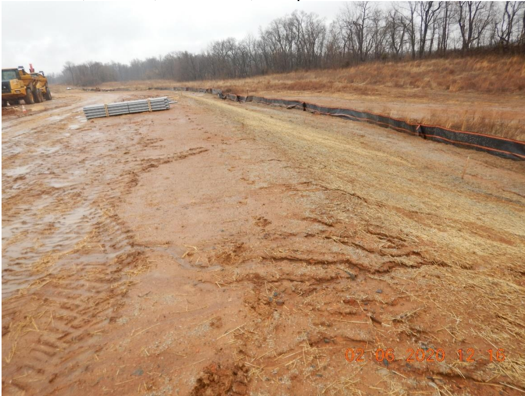
No fill slope protection on constructed slopes with erosion rills.
