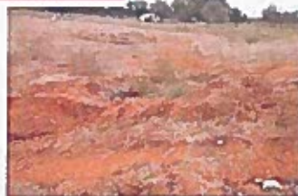
Two potential sinkholes pictured with earth berm protection in sediment basin #2.
