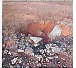
Sinkhole in basin #2.
