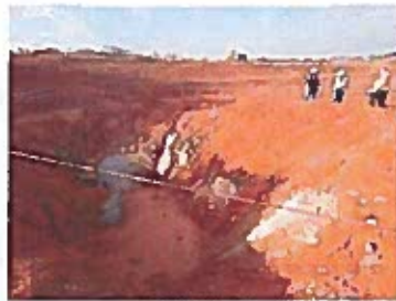
Sinkhole in Basin #1
