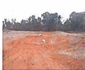
Overview of sinkhole in sediment basin #1.
