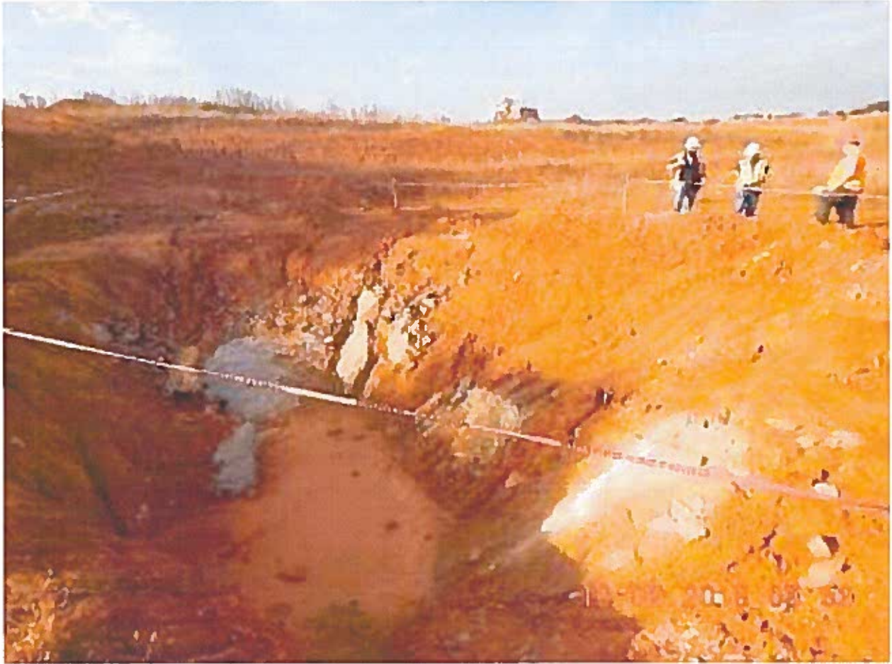
Sinkhole in Rockwool's Basin #1 – October, 2018
