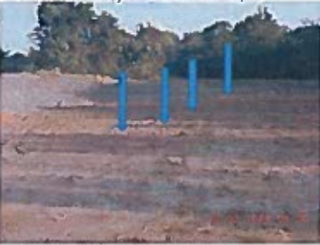
Four sinkholes pictured in the reuse pond.
