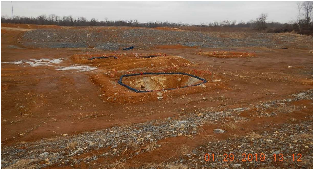
Figure 9. Several sinkholes in the Reuse Pond (WVDEP 2019a) with temporary structures to minimize the transport of sediment into the karst aquifer (photographer not named).
