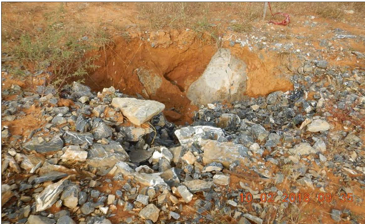
Figure 11. Sinkhole in Sediment Basin #2 (WVDEP 2018a) (photographer not named).
