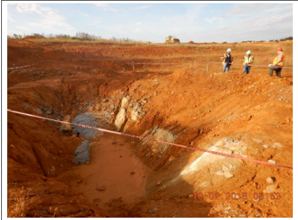
Figure 6. Closed depression or sinkhole in the RAN 5 facility Basin 1 (WVDEP 2018a). All of the rock and soil where the depression is now has moved down through fractures into solutionally-enlarged voids in the bedrock, and aquifer, beneath. This sediment is a contaminant in groundwater (photographer not named).
