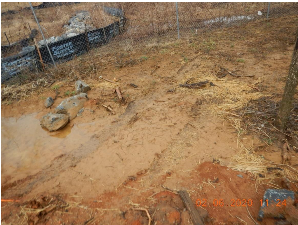
Sediment deposit outside the LOD below Sediment Basin. No perimeter controls installed at this location.
