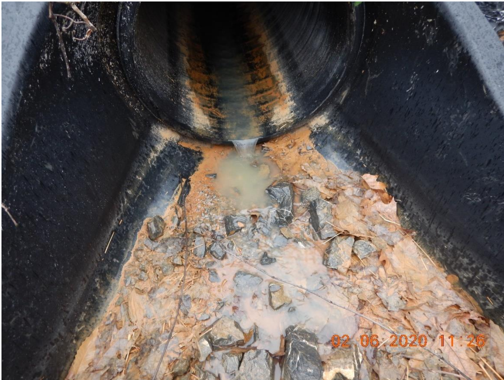
Sediment laden water coming out of sediment basin outfall.
