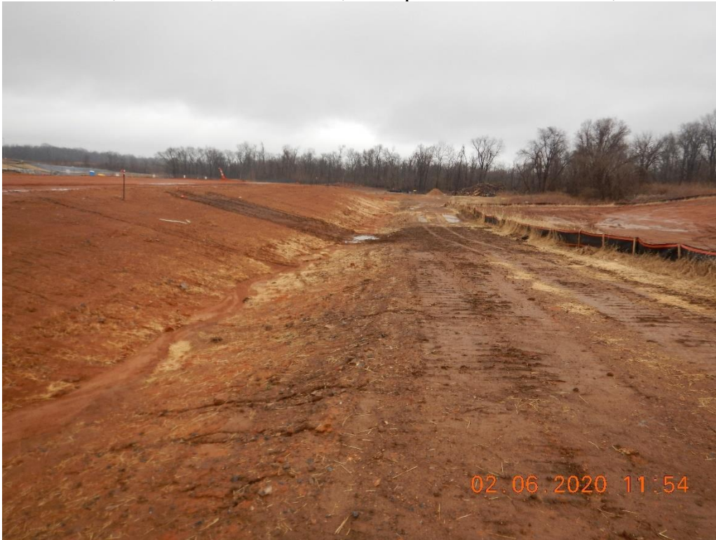
Diversion channel not installed per plan sheet details with ECM and rock check dams.
