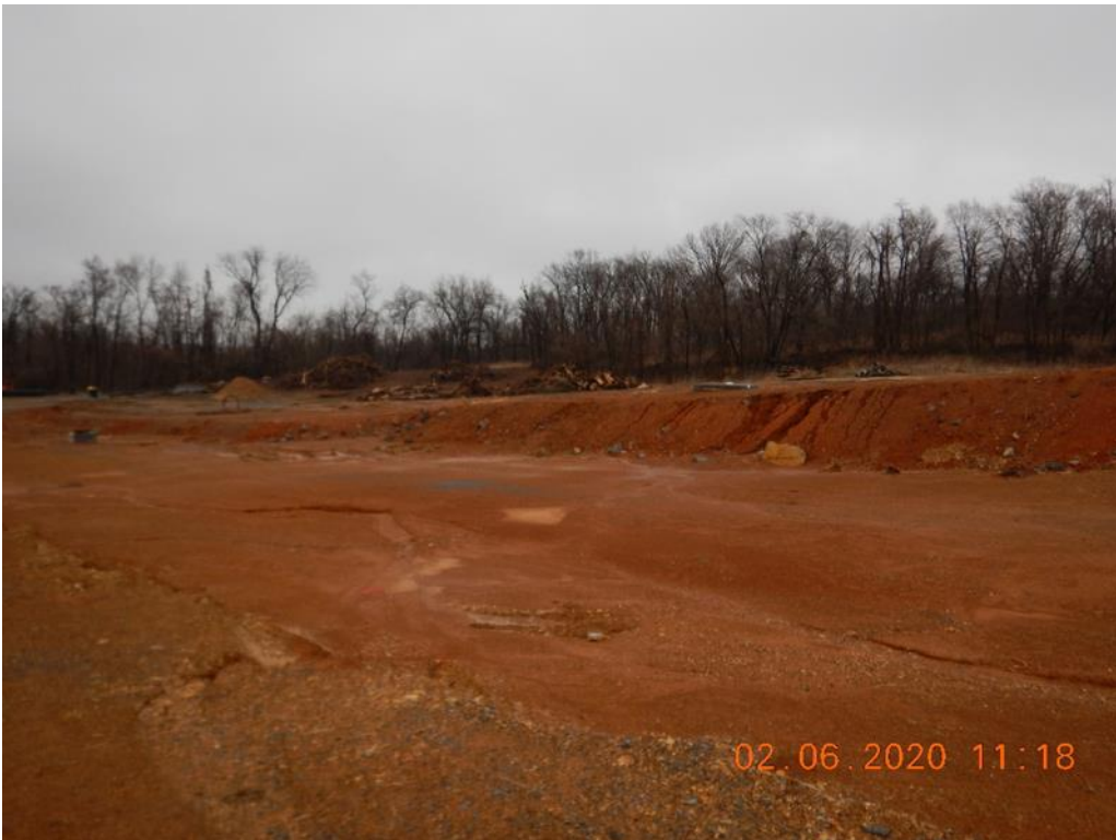
Soil stockpiles are not temporary stabilized with erosion rills.
