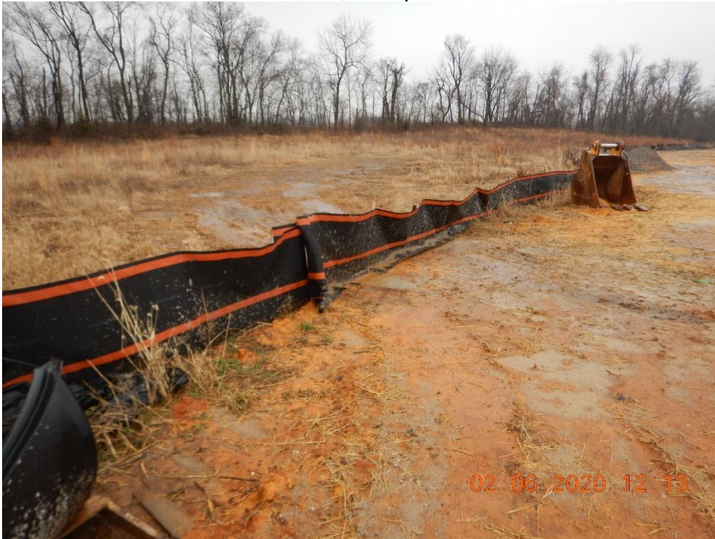
Multiple construction entrances along LOD of project that are not rocked.
