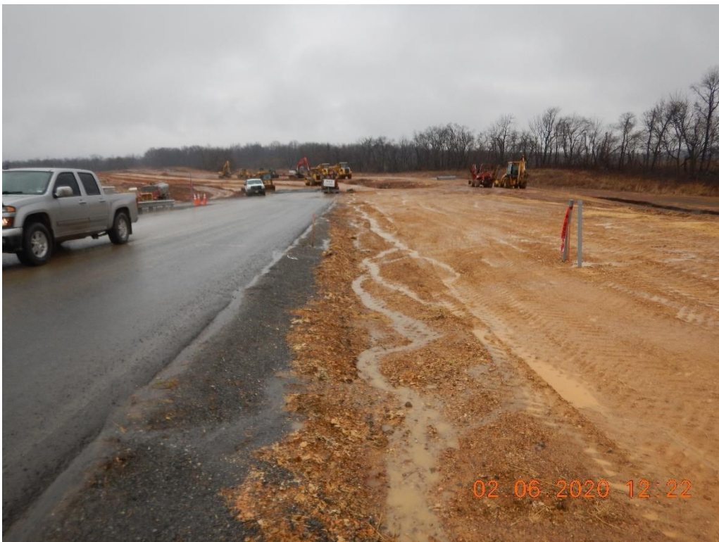
Diversion along Northport Ave. does not have rock check dams as indicated on plan sheet 9.
