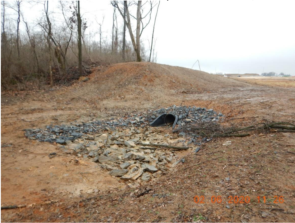
Outfall of sediment basin with not signage posited. Rip rap apron is stained with sediment from improperly operated basin.
