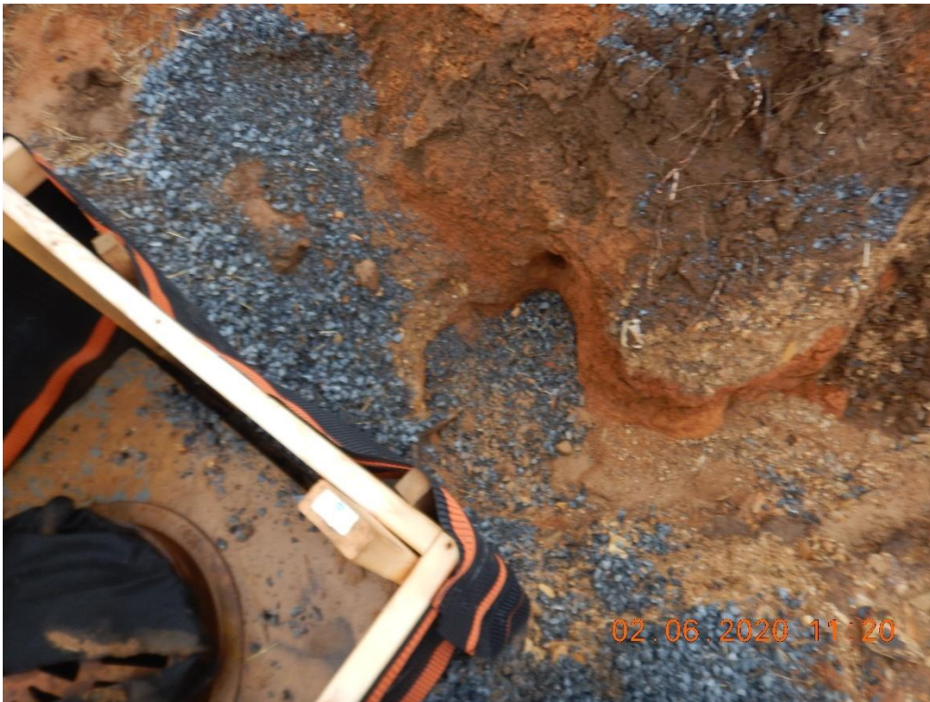
Maintenance on Drop Inlet protection where rock apron has been eroded away.
