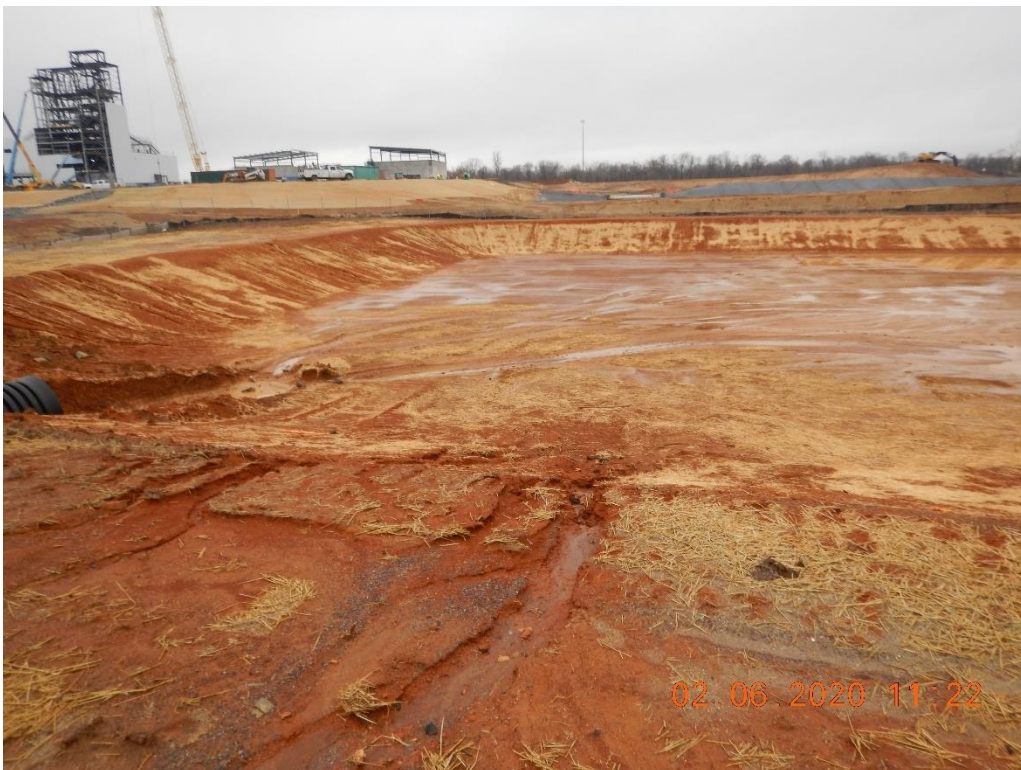
Unprotected inlets into sediment basin from erosion rills.
