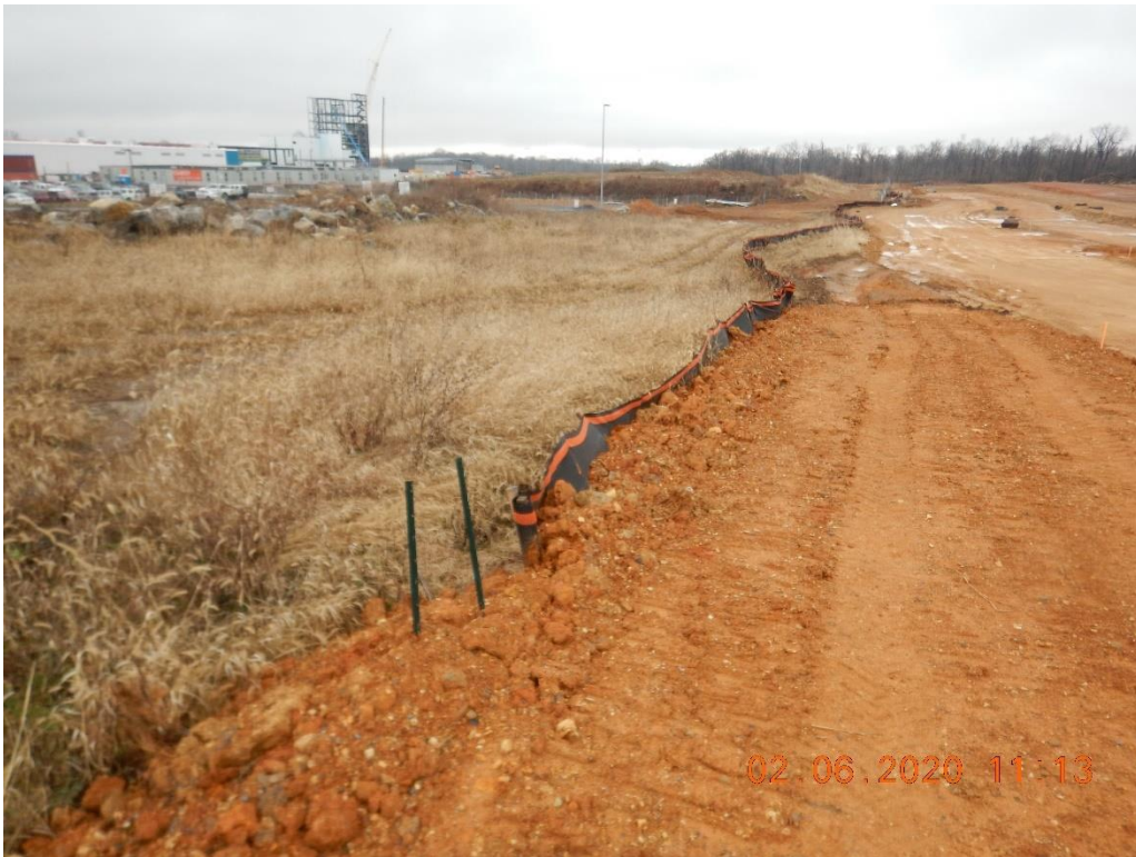
Where soil is being pushed up against silt fence, there is no holding capacity to allow proper filtration before being overtopped.
