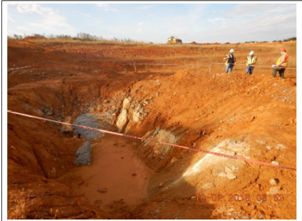
Figure 6. Closed depression or sinkhole in the RAN 5 facility Basin 1 (WVDEP 2018a). All of the rock and soil where the depression is now has moved down through fractures into solutionally-enlarged voids in the bedrock, and aquifer, beneath. This sediment is a contaminant in groundwater (photographer not named).
