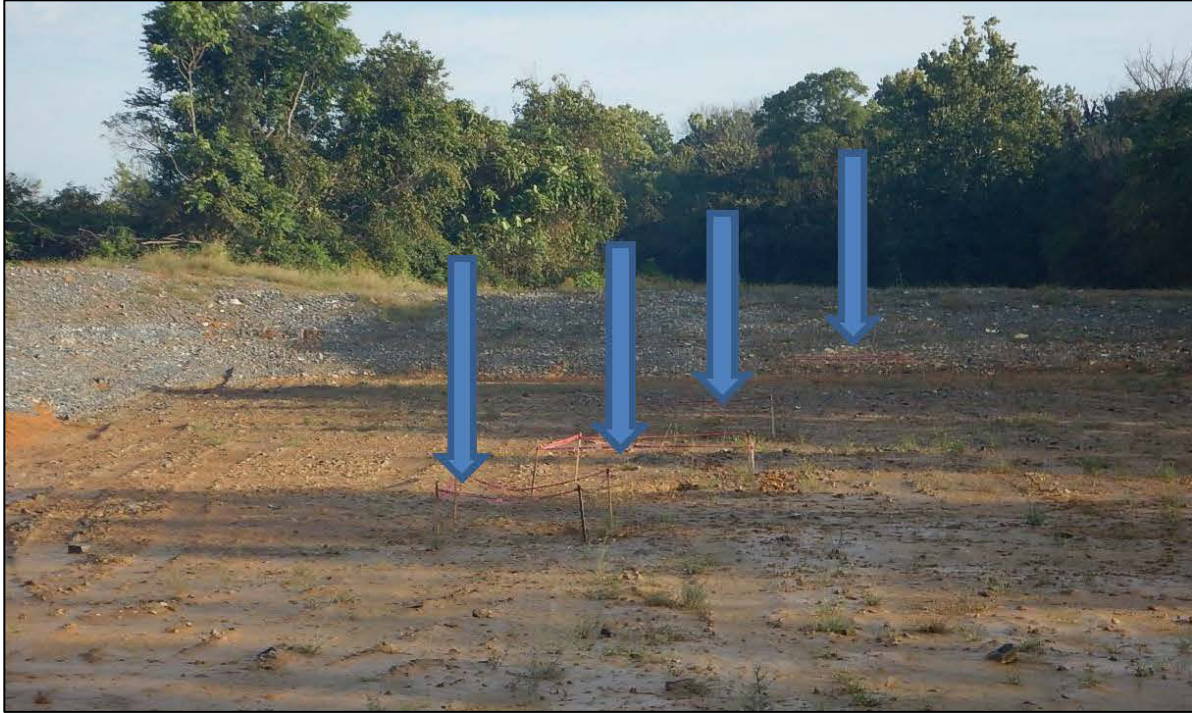
Figure 8. Four sinkholes in the RAN 5 Project Reuse Pond. (WVDEP 2018a) (photographer not named).
