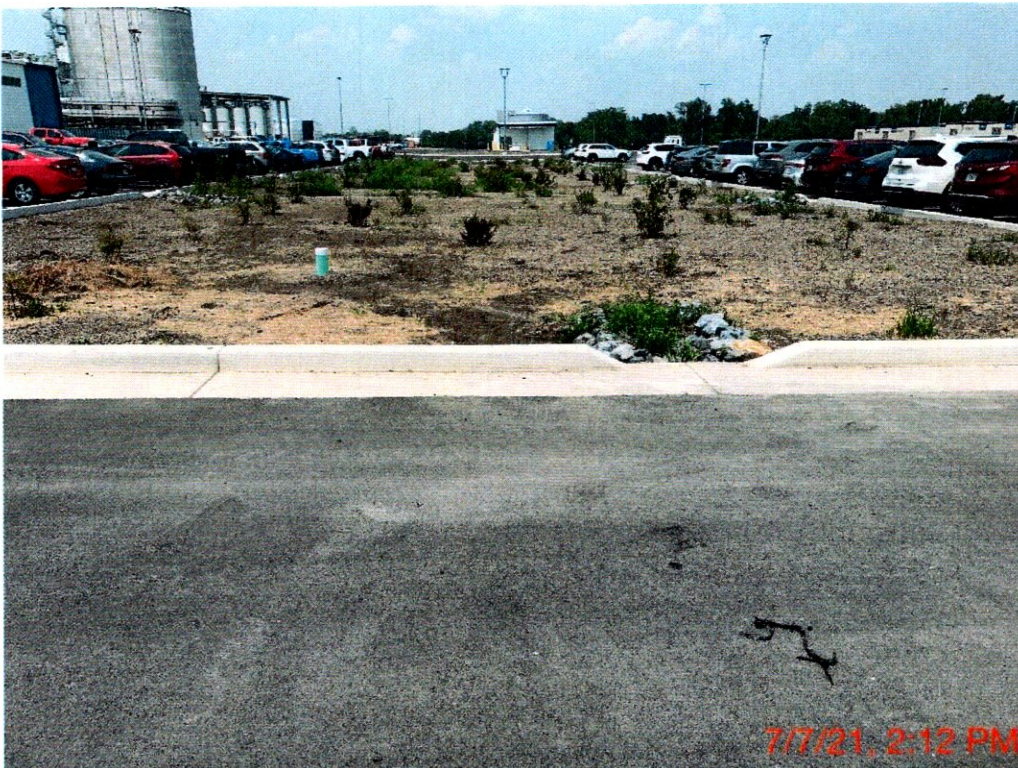
Bio Retention at the front parking lot
